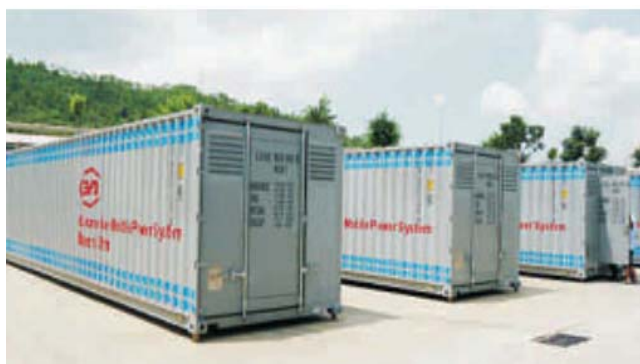
Figure 77: BYD's energy storage modular system
