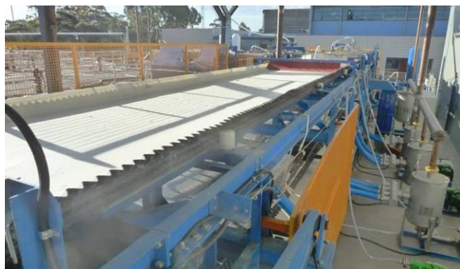
Figure 247: Rincon demonstration plant vacuum filter
