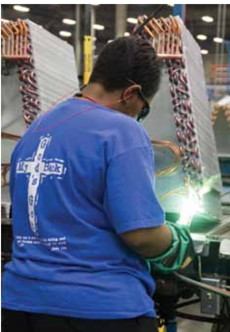
Tameka Black brazes distributor tubes onto a coil at Advanced Distributor Products, which makes coils for residential applications.
